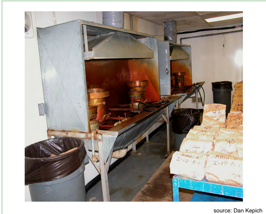
Figure 2-4-5 Fenwick Can Washers (Soil Sample Washing Machine) in Sample Wash Room
